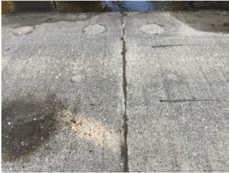
Cracking deck joint
